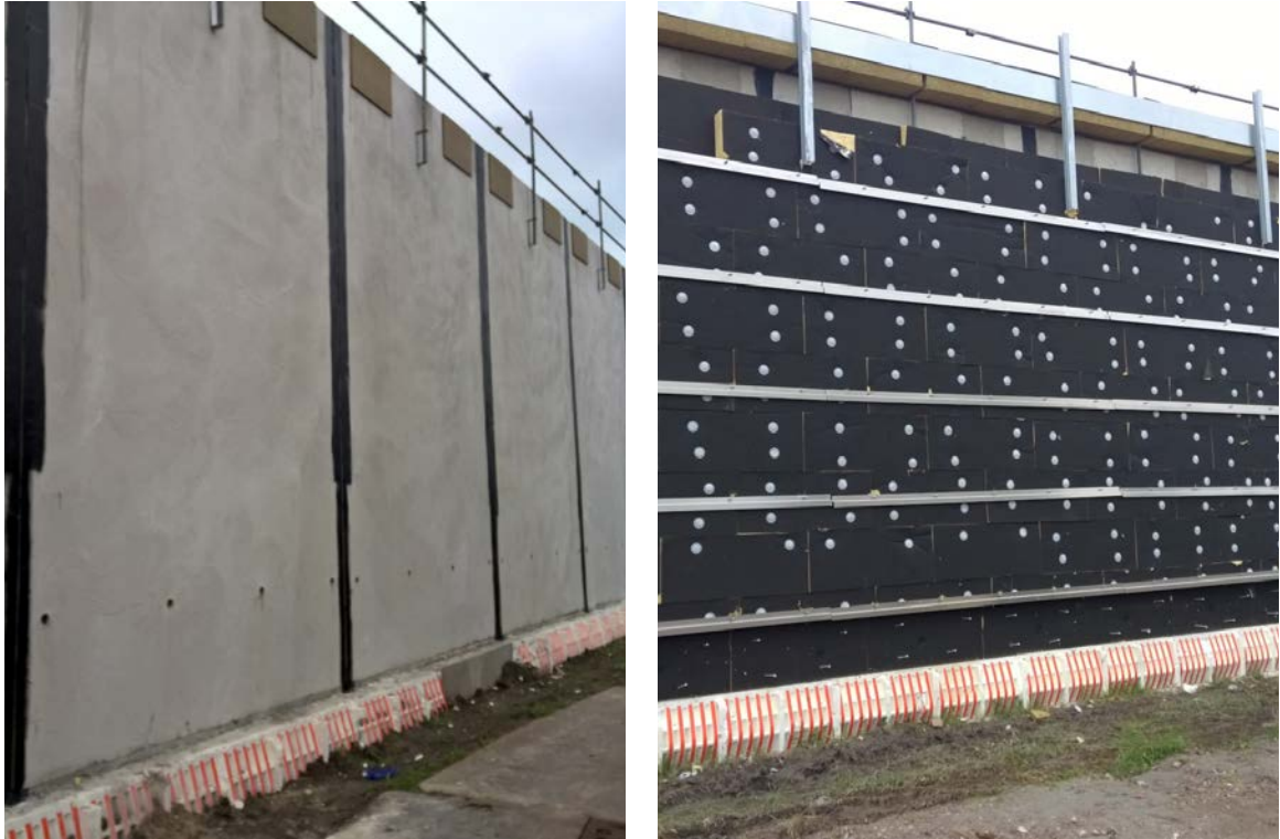
Figure 2 On the left the building constructed from prefab concrete and on the right the insulated outer shell. Photos: Luc Schaap
