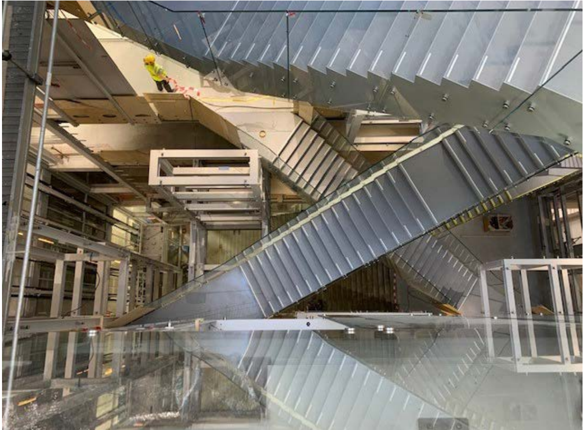
Figure 3 The stairwell during construction (left) and after completion and installation of art (right). Photos: Museum Boijmans Van Beuningen
